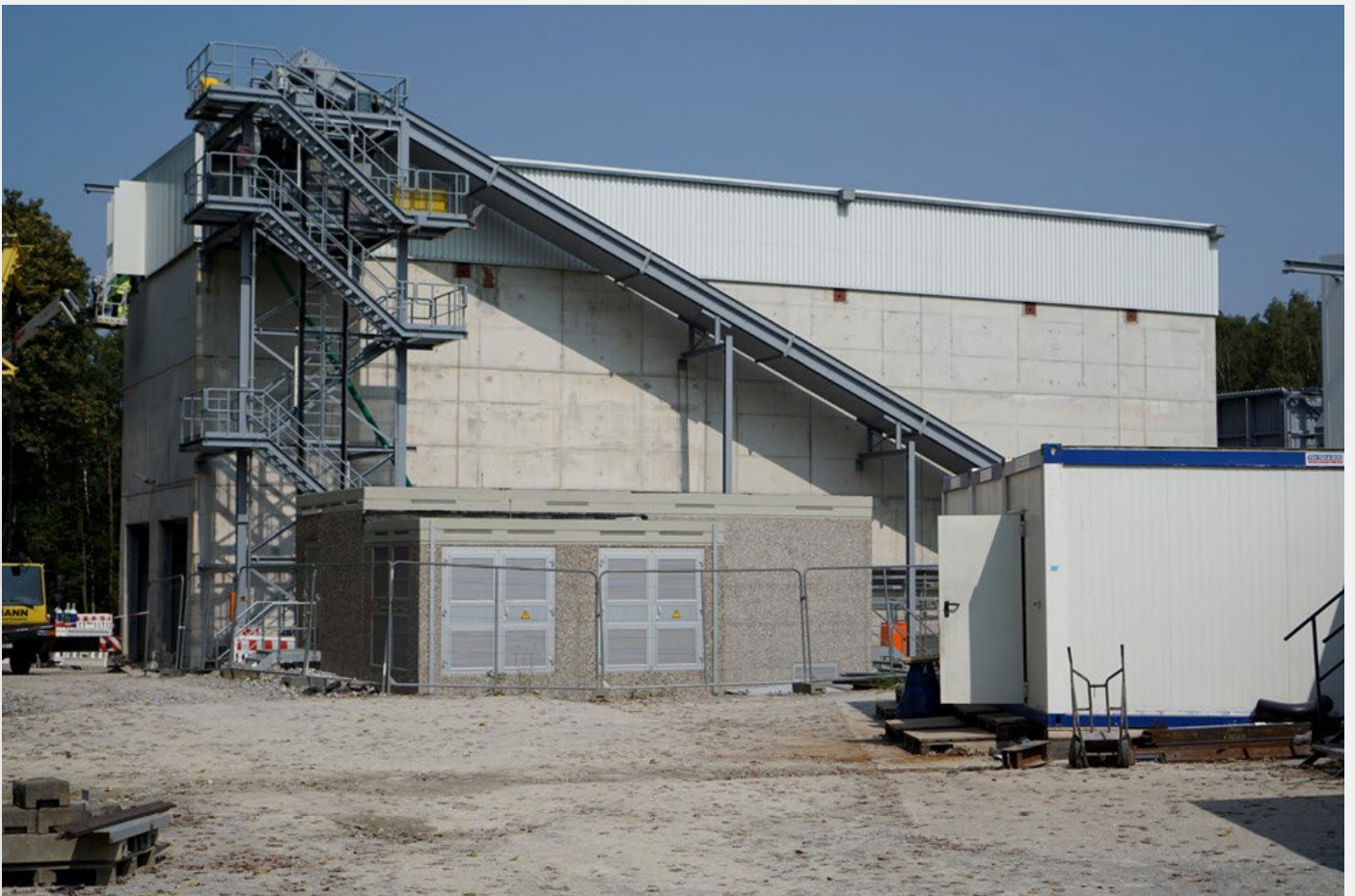
AF (alternative fuel) storing with automatic reclaimer
