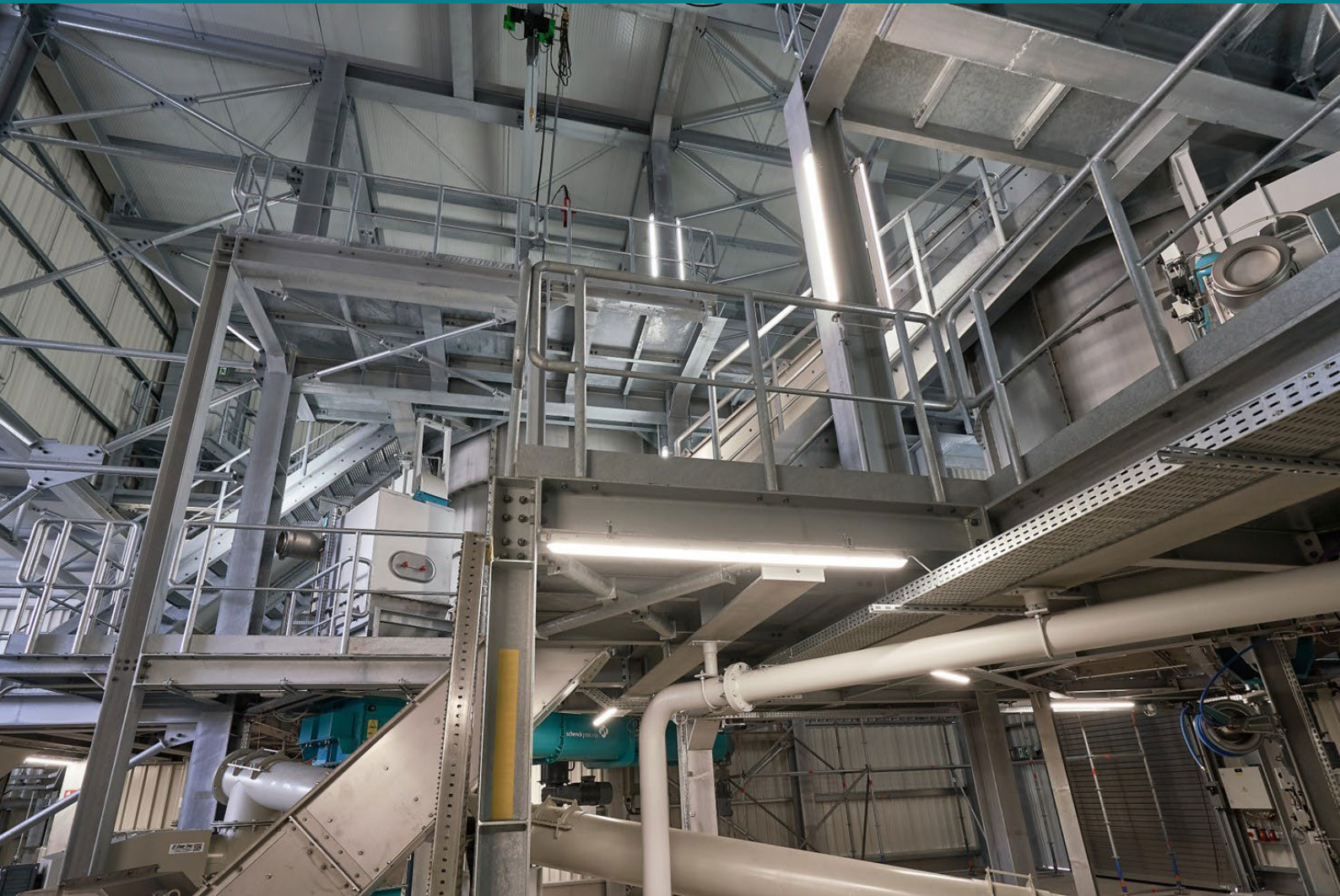
Installation dosing unit
