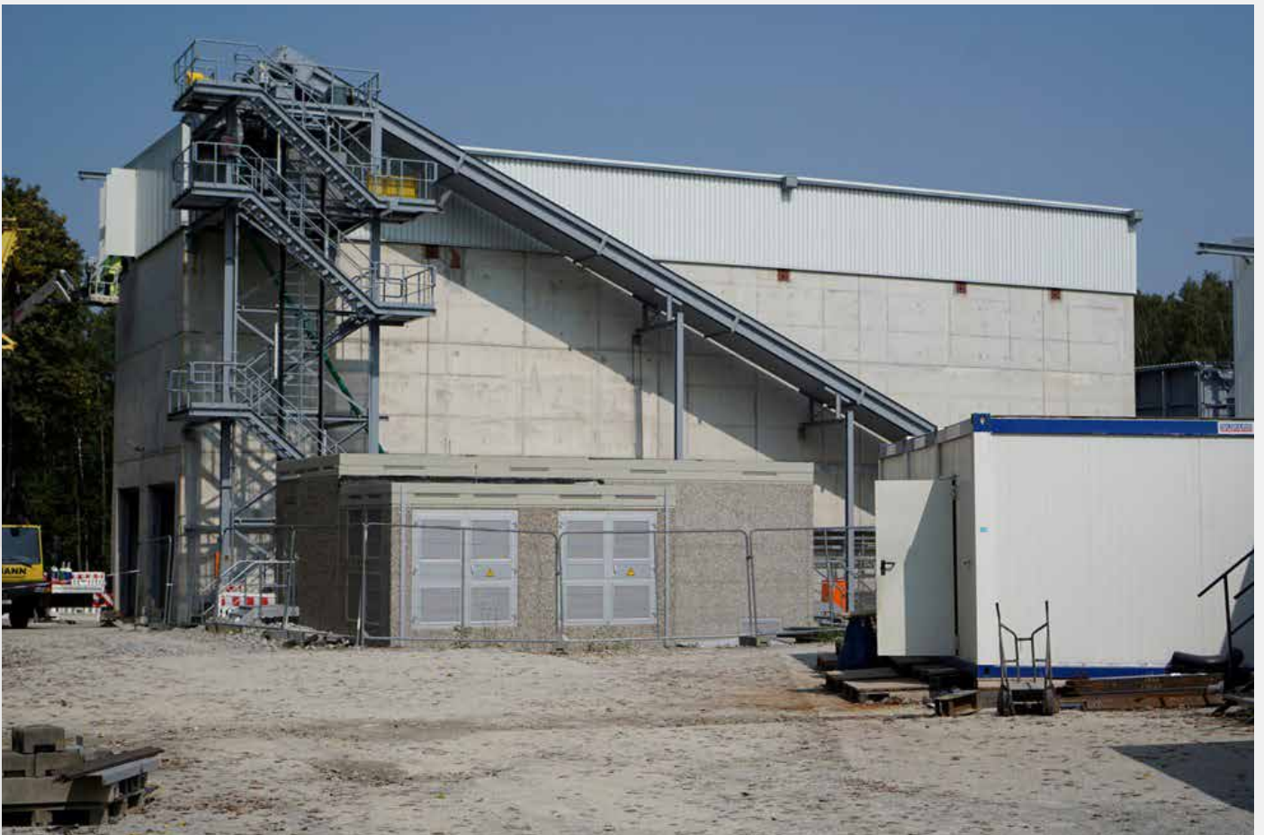
AF (alternative fuel) storing with automatic reclaimer
