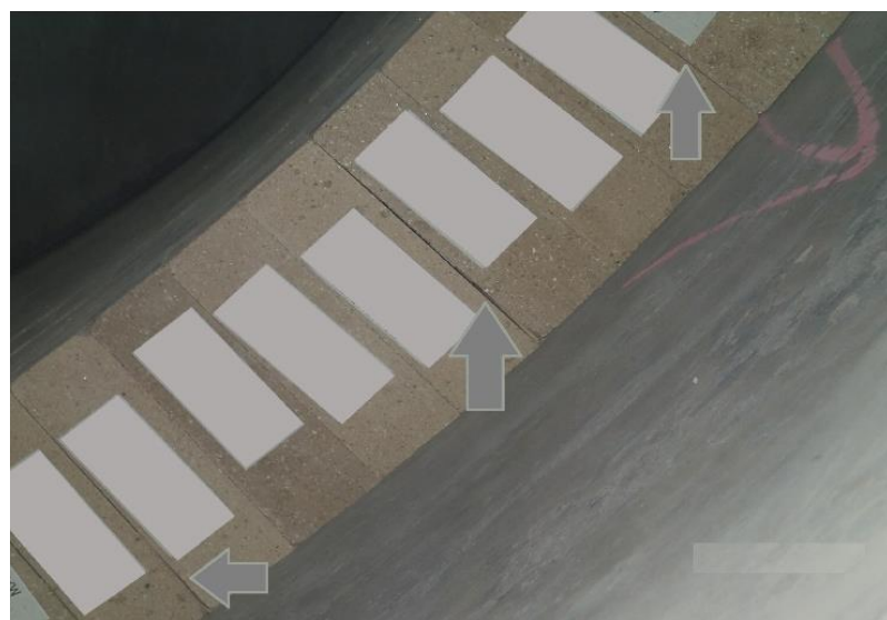
Figure 1: View of alumina brick showing varying size gaps between bricks
