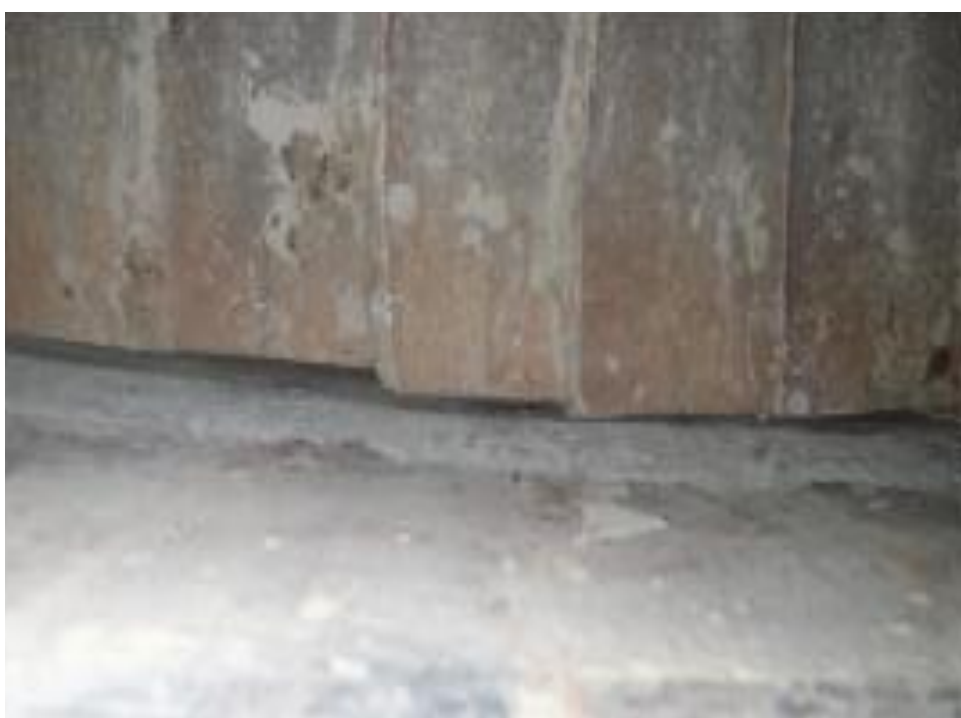
Figure 9: Stepping at base of bricks
