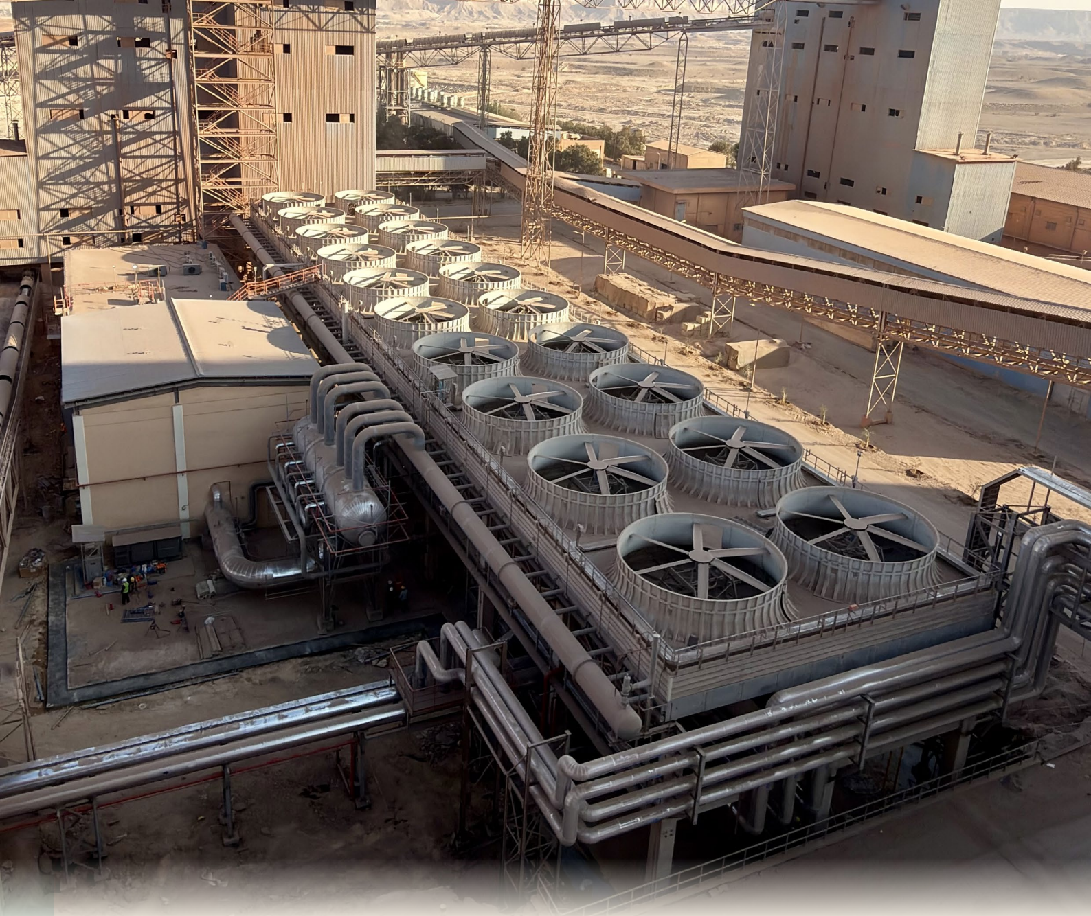
Turboden ORC in a cement plant, details of the ACC
