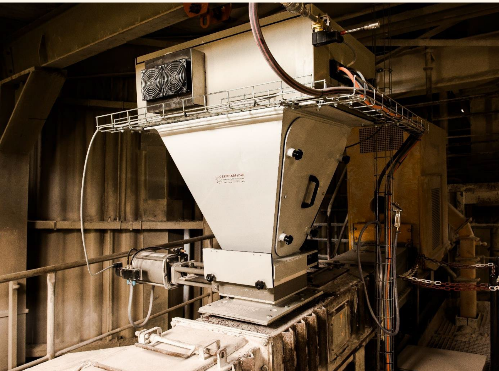
Figure 1 - SpectraFlow Online NIR Airslide Analyzer fitted to an airslide in a cement plant.
