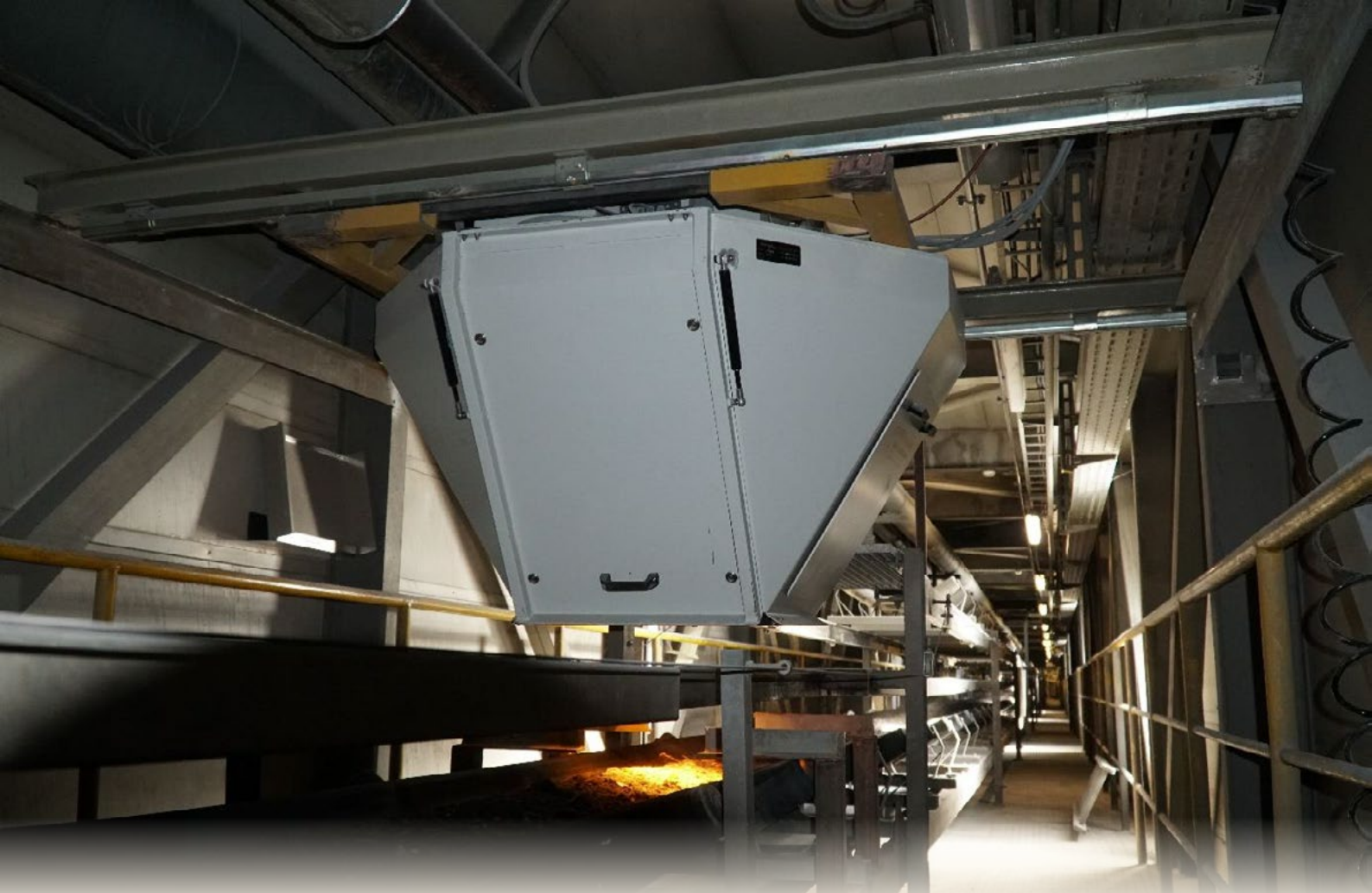
Figure 2 - SpectraFlow Crossbelt Analyzer installed over a conveyor belt for raw material measurement.
