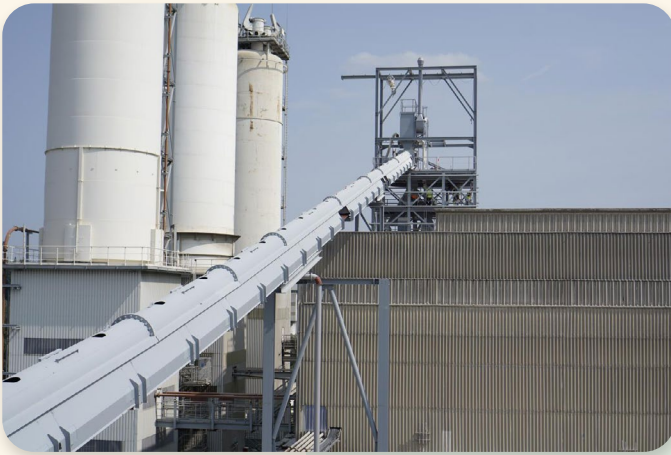
5. Air-supported belt conveyor
