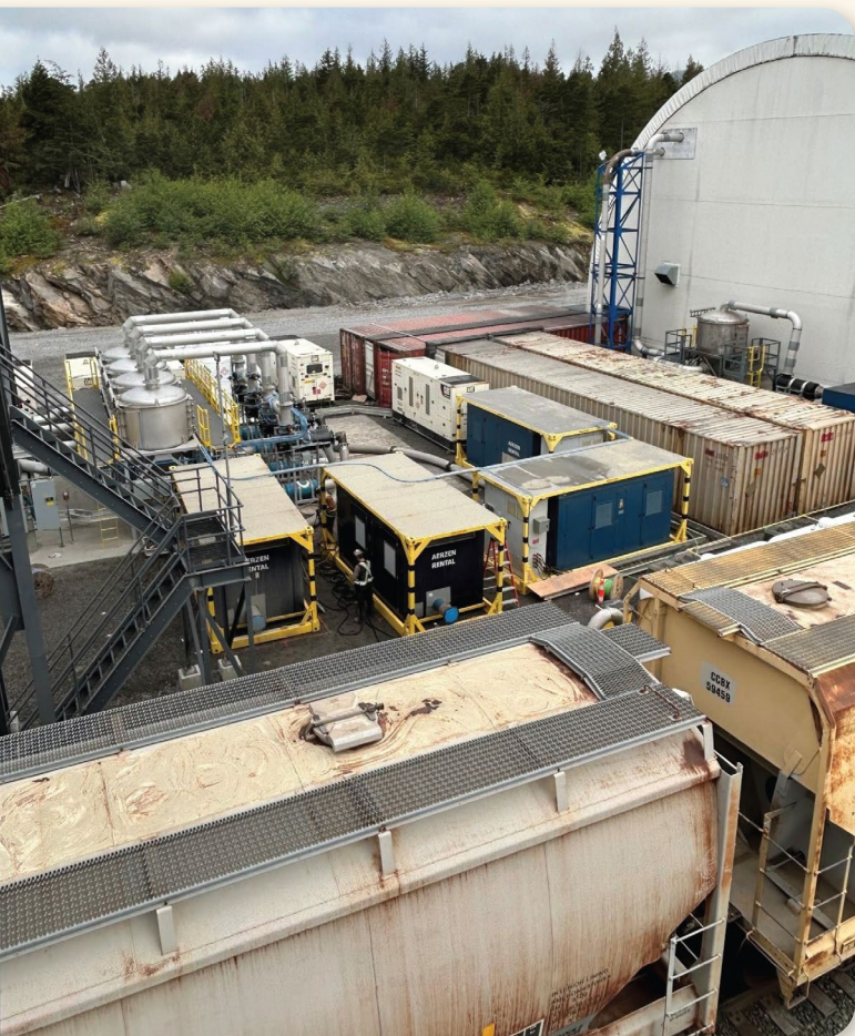
Figure 3. Rental Process Blowers at a Repackaging Plant Startup in Canada
