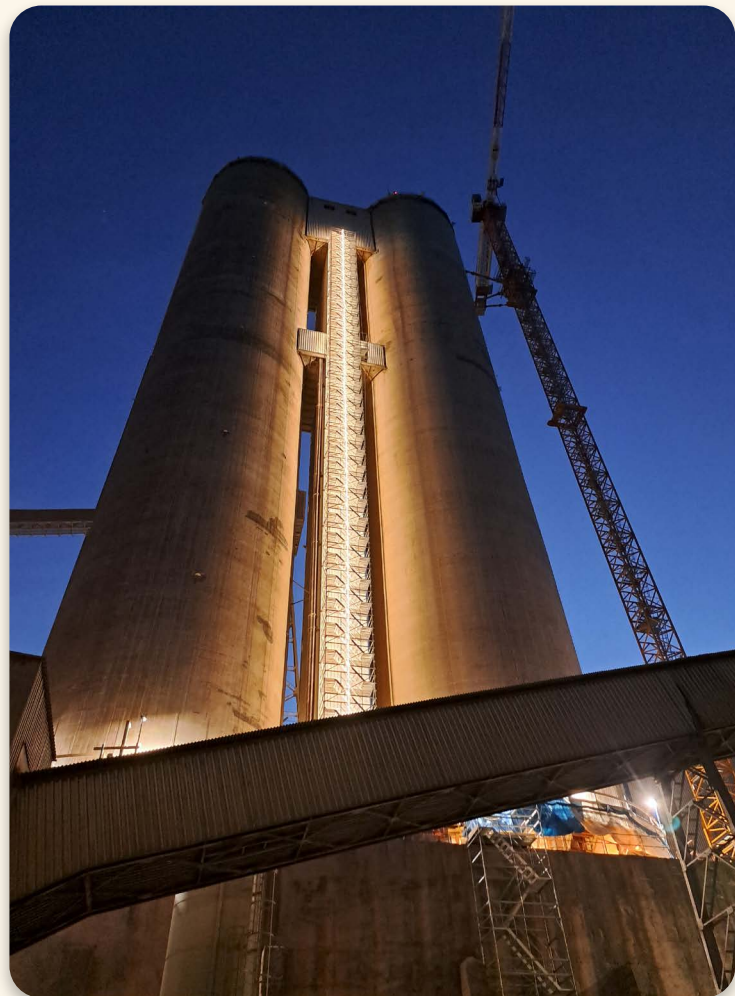
Old silos before repair
